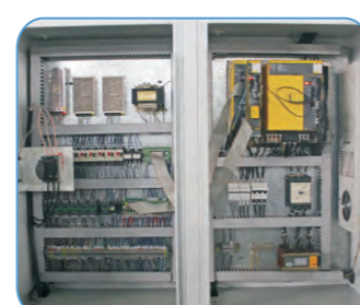
CE Norms Electric Cabinet
